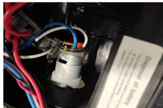
Step 5. Check the motor connection
