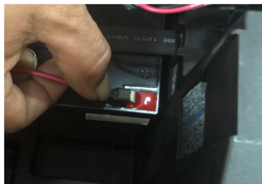
Step 3. Check the battery cable connection
